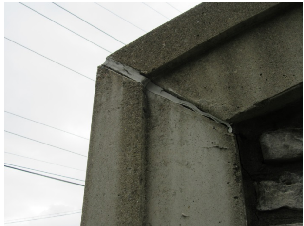
Adhesive and cohesive sealant failure at entrance monument
