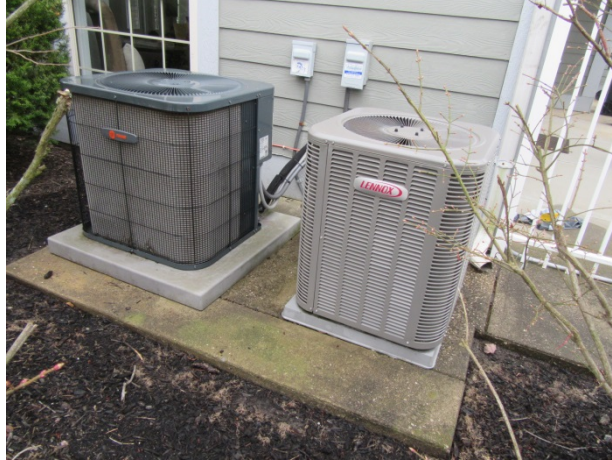
Condensing unit overview
