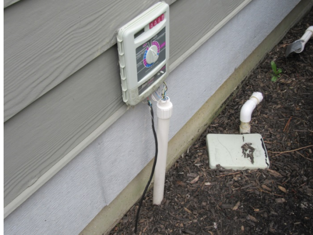
Exposed wiring and control panel
