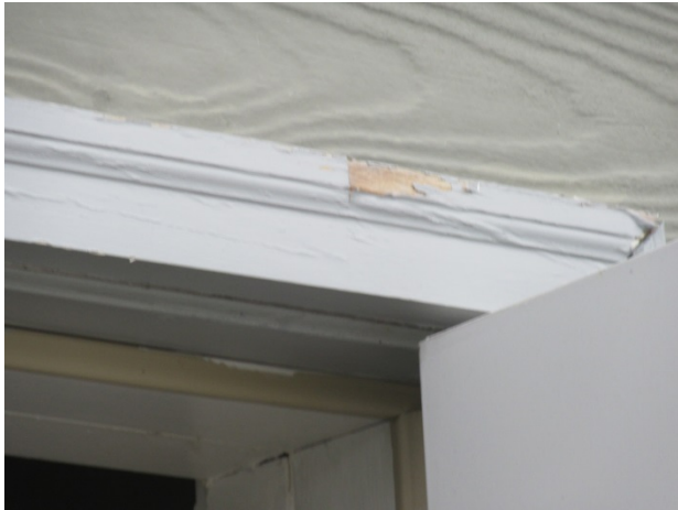
Paint deterioration above rear door
