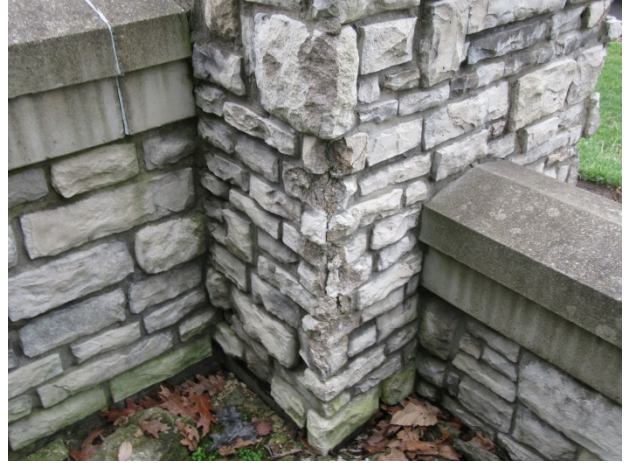
Cracks and deterioration at entrance monument
