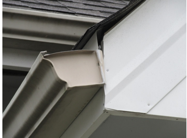
Lifted apron at rear
