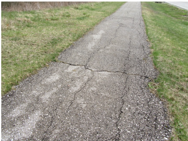
Cracks near Turfrider Court
