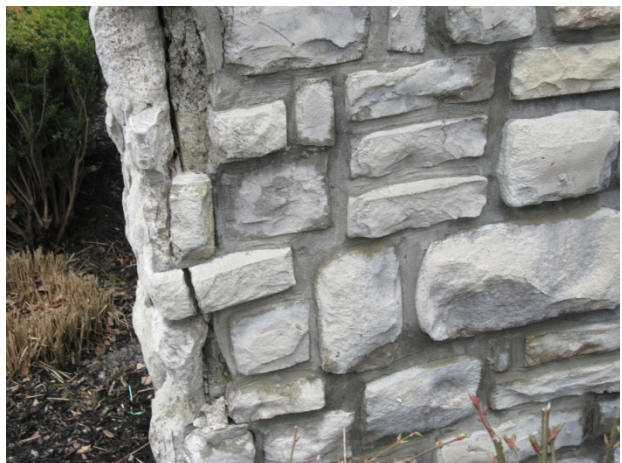
Cracks and deterioration at entrance monument
