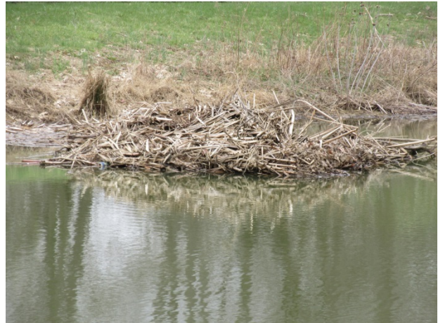
Debris accumulation at western pond control structure
