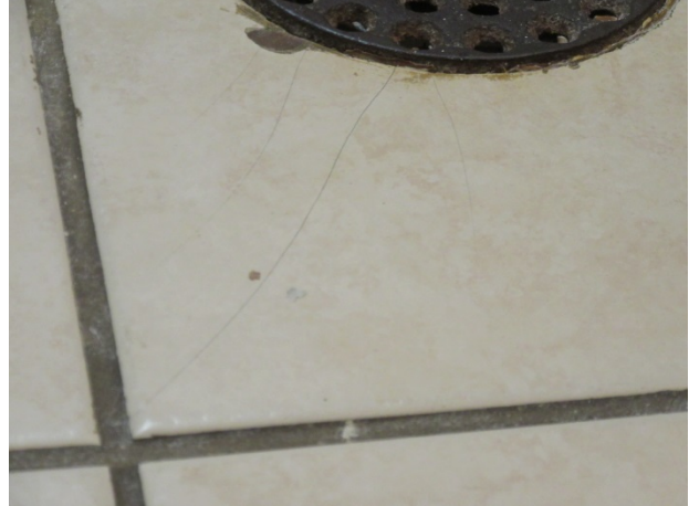
Cracked tile in rest room
