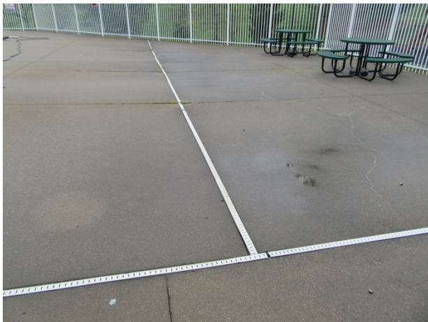
Crack repairs and organic growth
