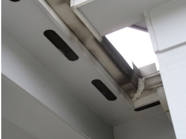
Discoloration at rear
