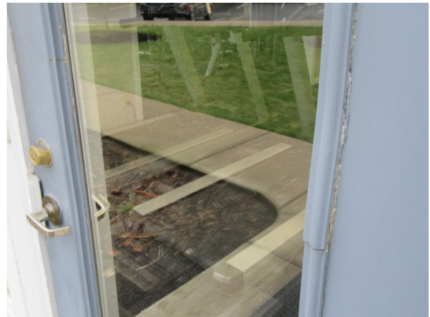
Gym door frame deterioration
