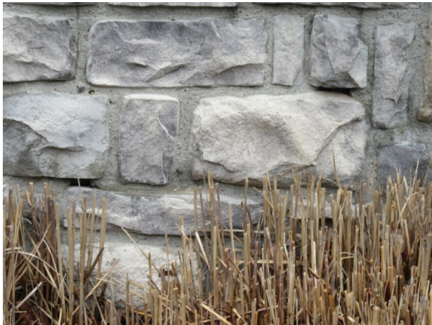
Clubhouse signage mortar deterioration
