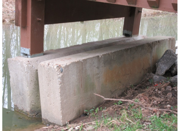
Settlement of concrete footing
