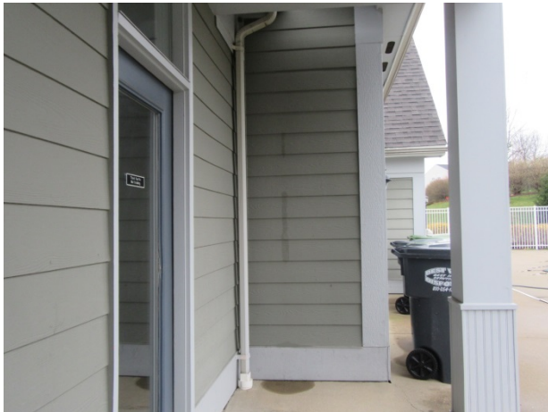
Overflow at rear
