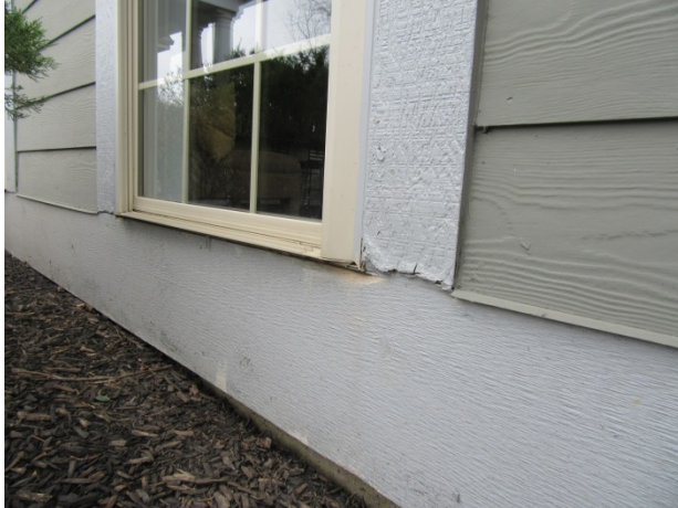
Wood rot at western side
