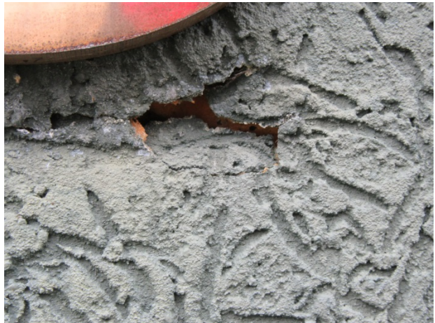
Clubhouse signage damage
