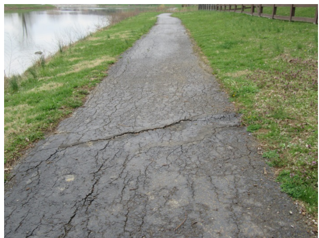
Cracks north of central pond
