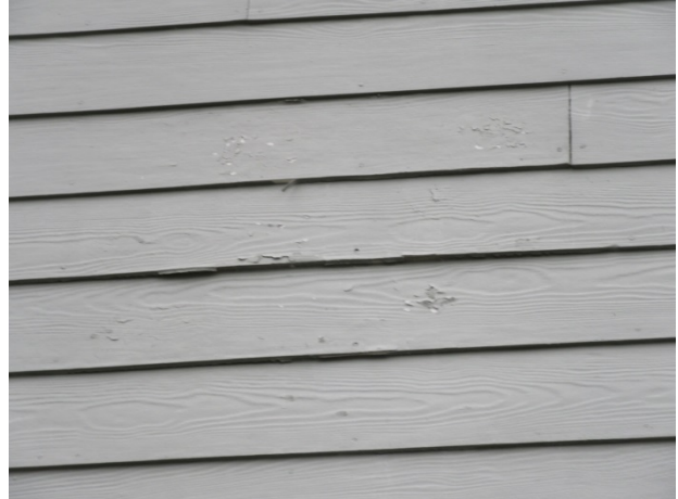
Paint deterioration at western side
