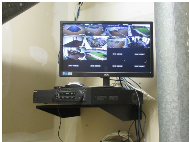
Recorder and monitor overview
