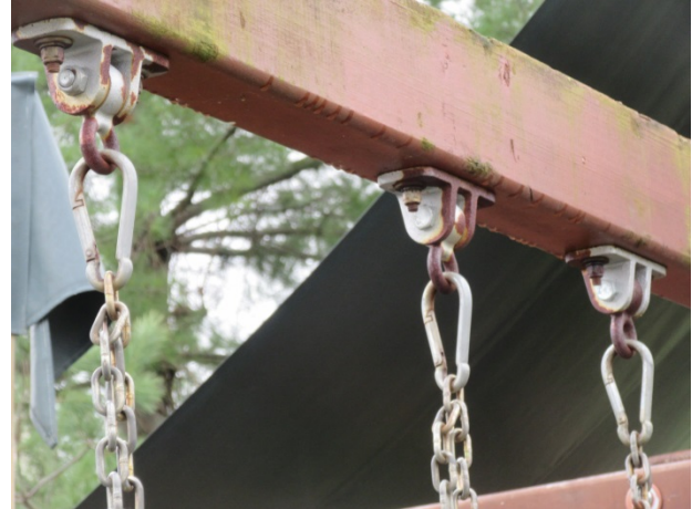
Rust and organic growth
