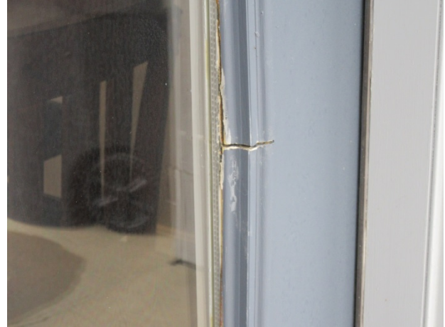
Rear door frame deterioration
