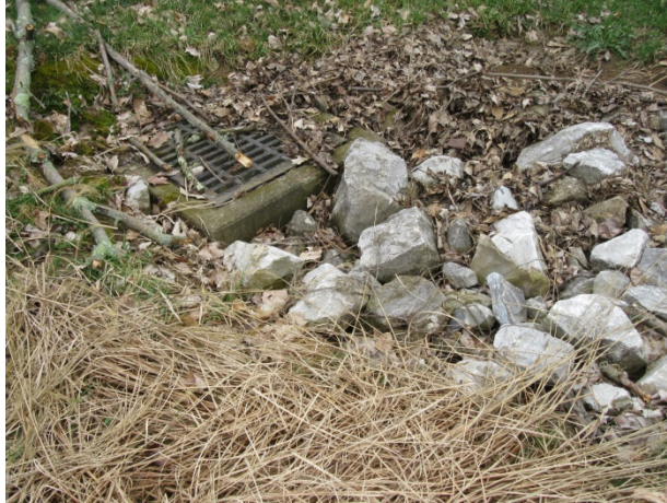
Catch basin near southeastern end of Foxhunt Drive
