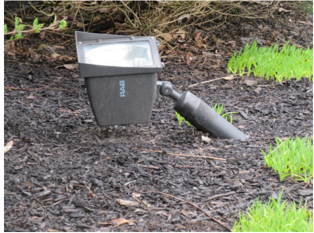
Displaced light fixture
