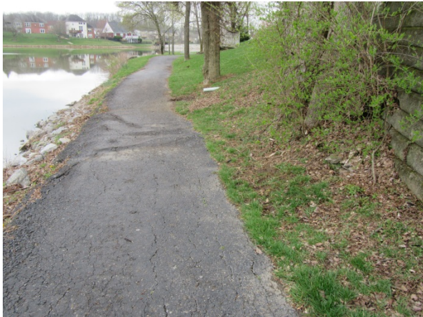
Cracks and upheaval due to tree roots northwest of central pond
