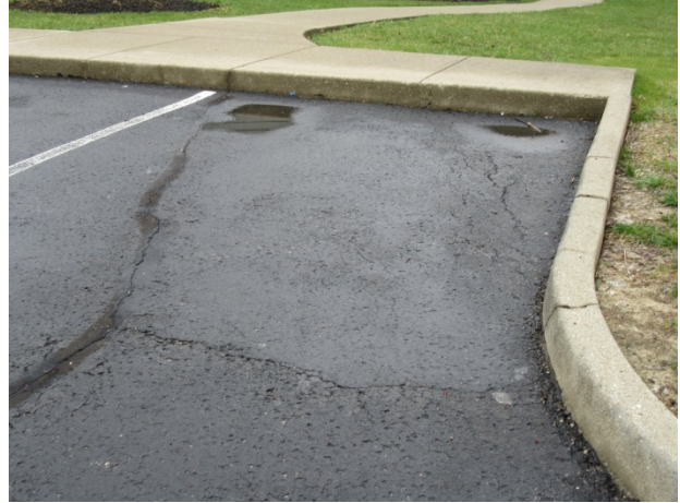
Tire ruts and cracks
