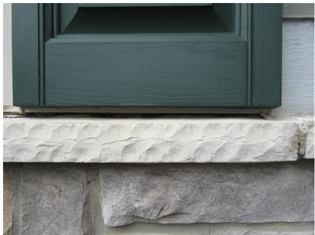
Missing sealant and potential for water accumulation
