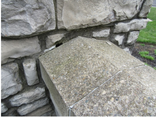
Deterioration and potential for water infiltration at entrance monument
