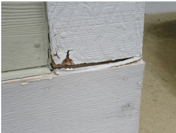
Wood rot at rear
