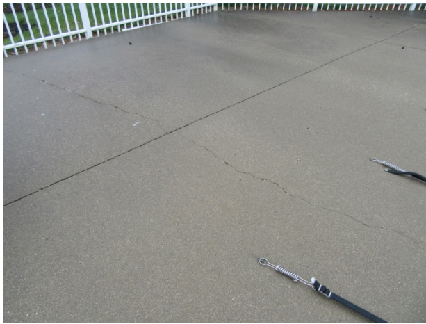
Pool deck crack
