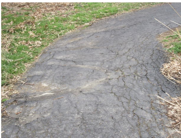
Alligator cracks and uneven pavement north of central pond
