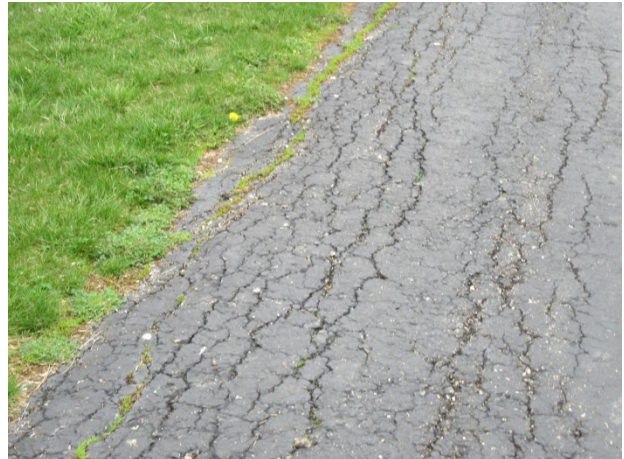
Alligator cracks and organic growth west of central pond
