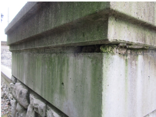
Entrance monument mortar deterioration
