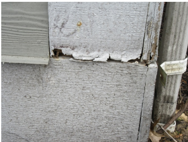
Wood rot at front
