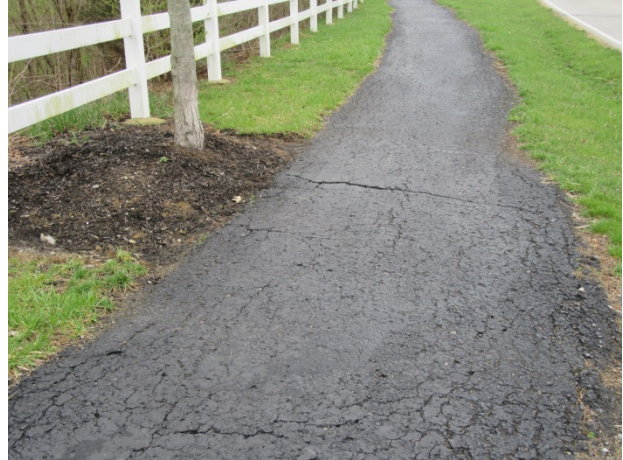
Crack likely due to tree root near clubhouse
