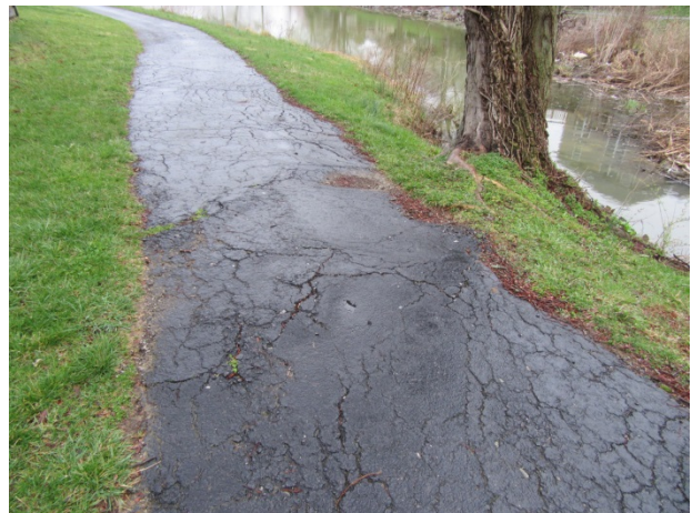
Alligator cracks and upheaval due to tree roots near northern bridge
