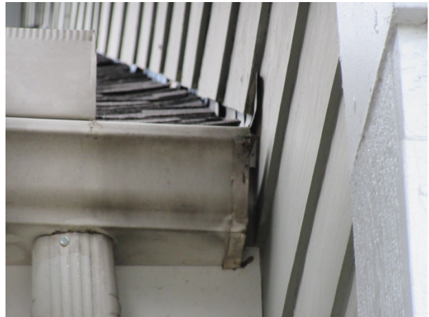
Displaced gutter (cause of overflow)
