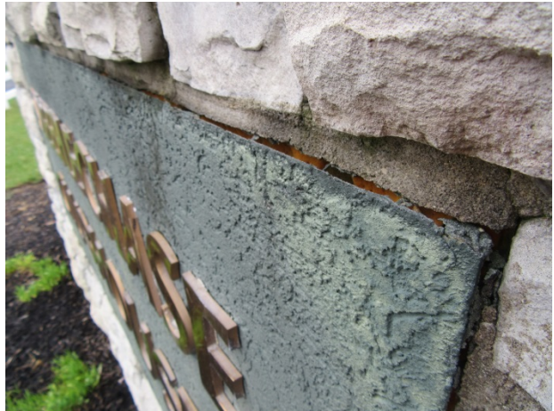
Separation and potential for water infiltration
