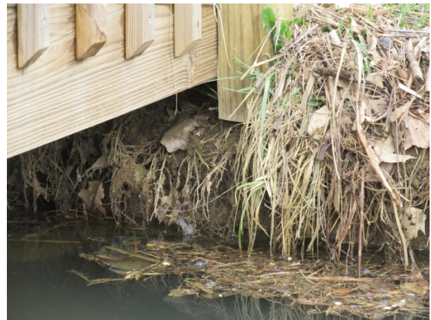
Support on eroding shoreline
